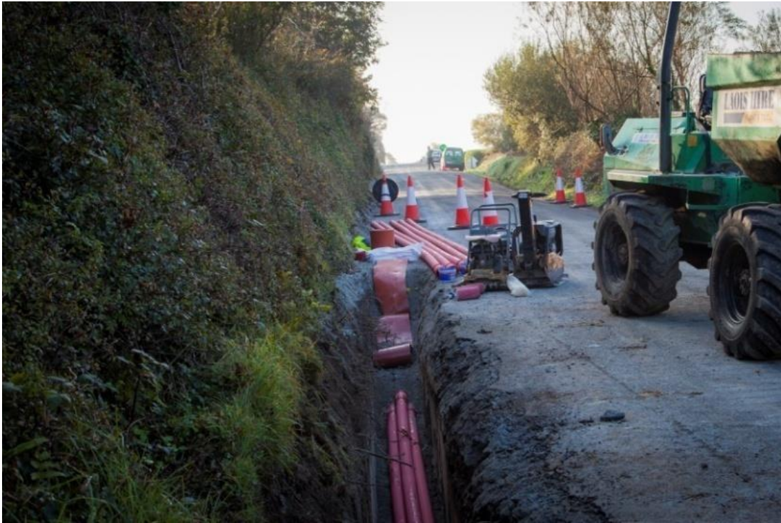
Figure 3-24 Typical ducting installation works for a grid connection cable trench on public road
