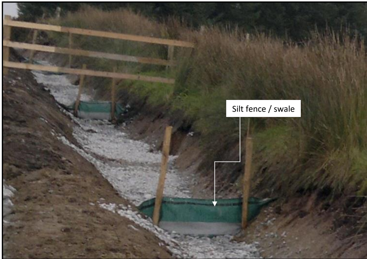
Figure 3-38 Example of a silt fence used in conjunction with check dams along roadside drainage channels
