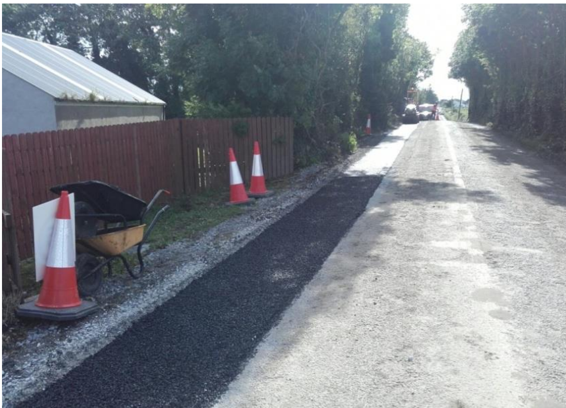
Figure 3-25 Typical permanent reinstatement works for a grid connection cable trench on public road
