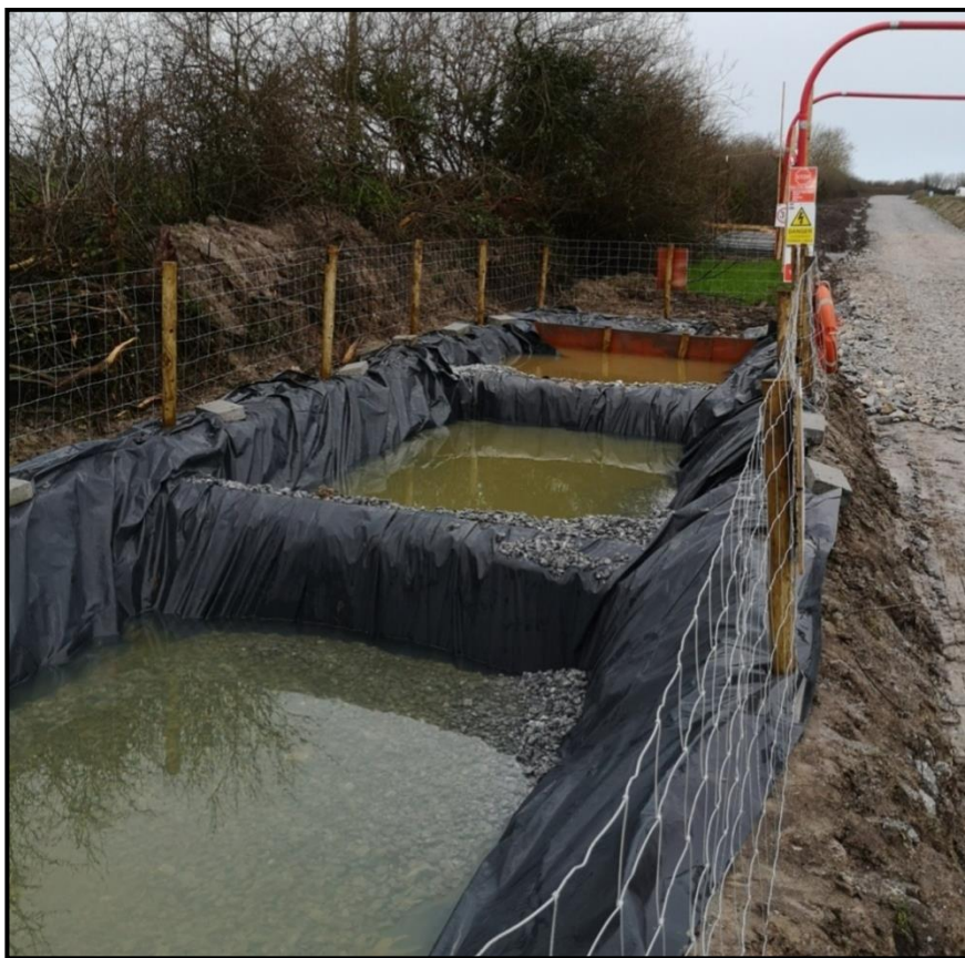
Figure 3-36 Multi-tiered settlement pond with stone filter
