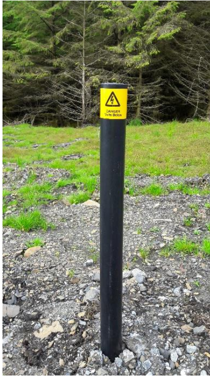
Figure 3-22 Example of a typical cable marker post on a wind farm
