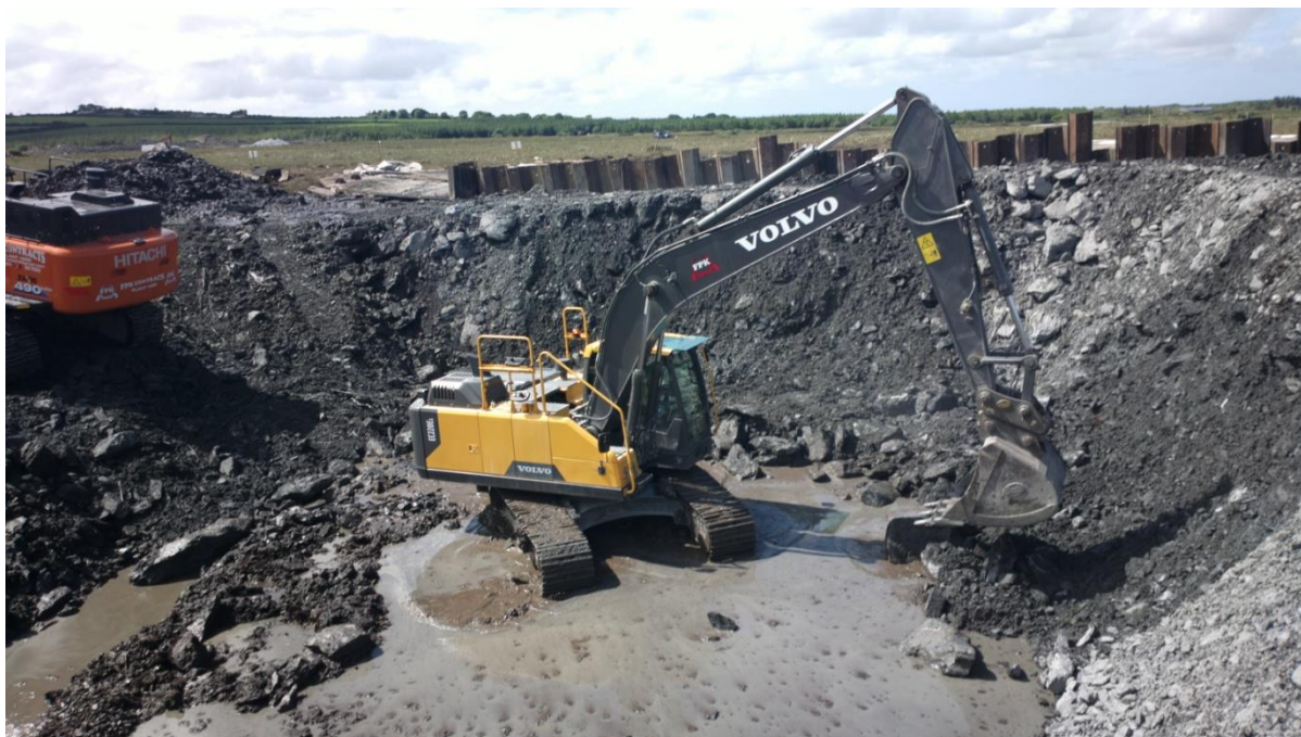
Figure 3-18 General Excavation towards the centre after fill is placed beside the sheet piles
