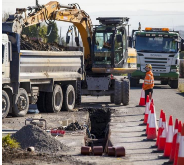
Figure 3-23 Typical excavation works for a grid connection cable trench on public road
